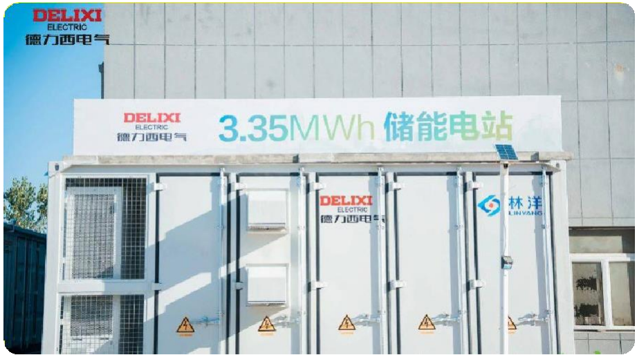
Energy Storage Station
